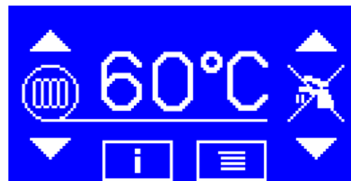
HEATING OF DHW OFF
